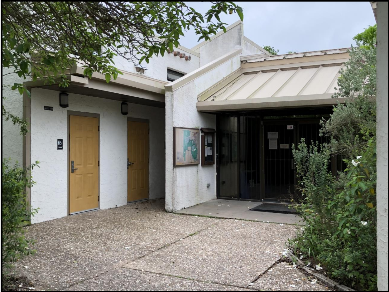
The restroom sign needs to be larger, and the opportunities on the dividing wall changed.
